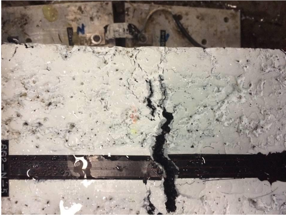
Fig 4 North section surface crack reached the inner vertical edge
